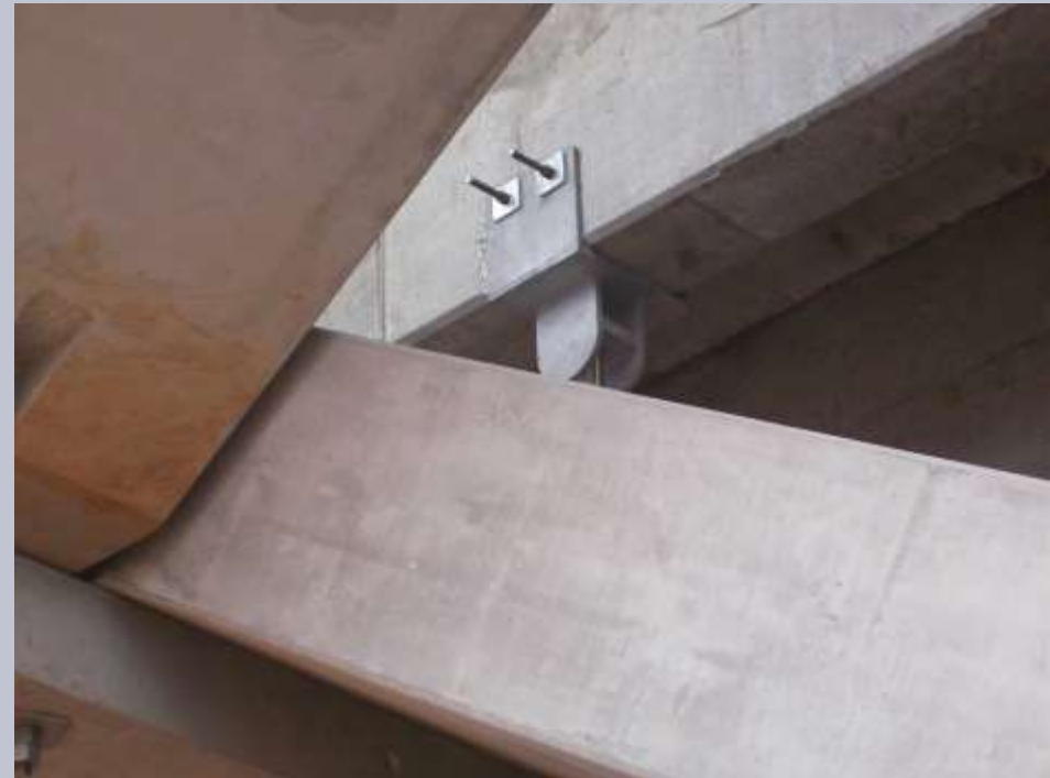
HOLE OMITTED – RETROFIT BRACKET FOR ROD
