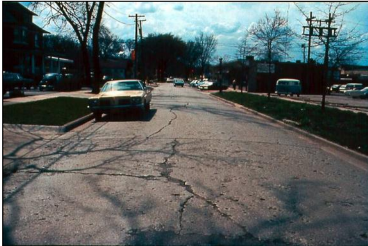
Erratic crack patterns due to no joints
